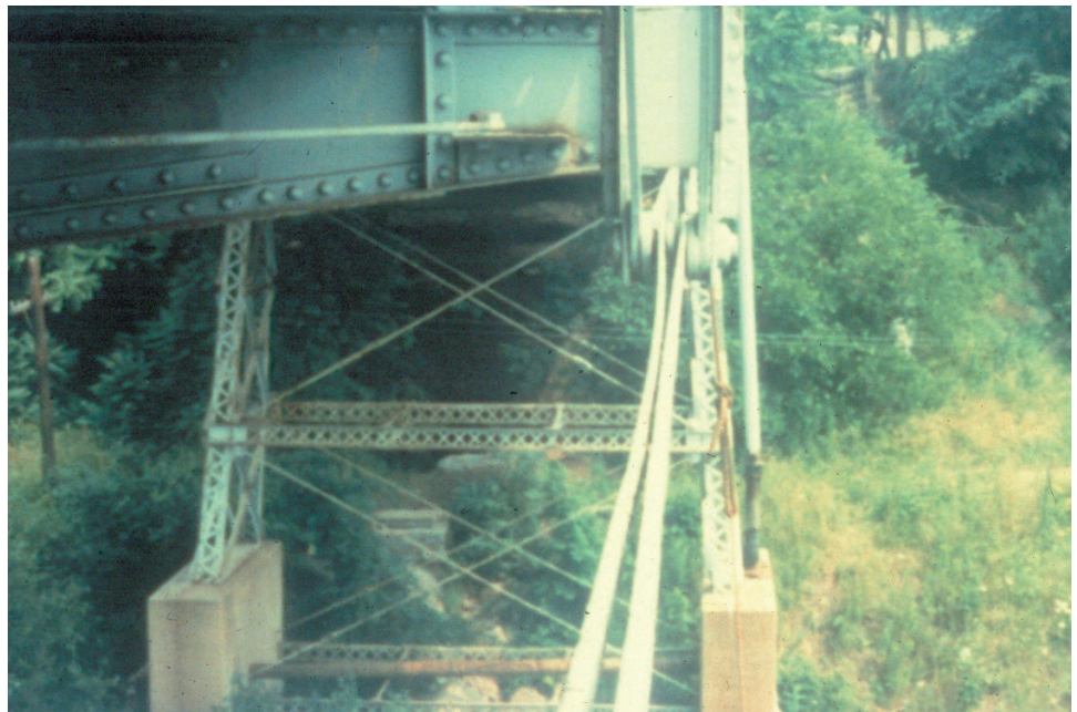
Figure 8.6.49 Bowed Bottom Chord Eyebar Member
