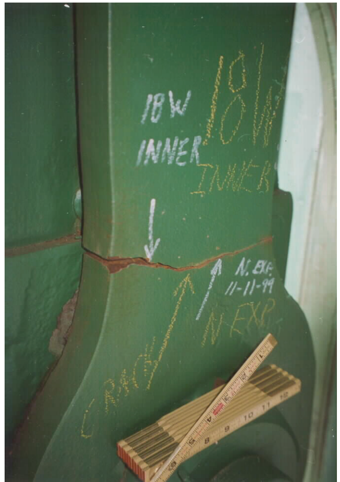
Figure 8.6.45 Cracked Forge Zone on an Eyebar
