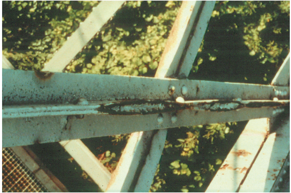
Figure 8.6.66 Sway Bracing with Rust Packing
