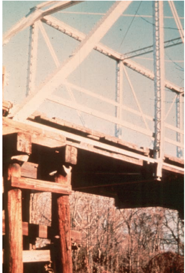
Figure 8.6.52 Buckled End Post and Temporary Supports
