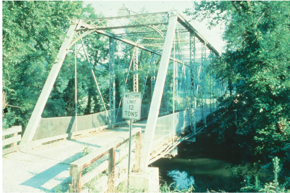
Figure 8.6.50 Buckled Lowered Chord Member L0L1, due to Abutment Movement
