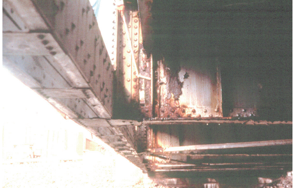
Figure 8.6.53 Corroded Floorbeam End and Connection
