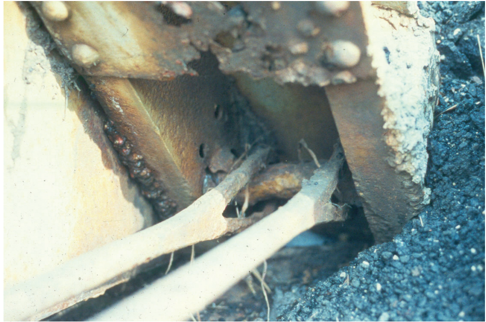
Figure 8.6.63 Worn and Corroded Pin
