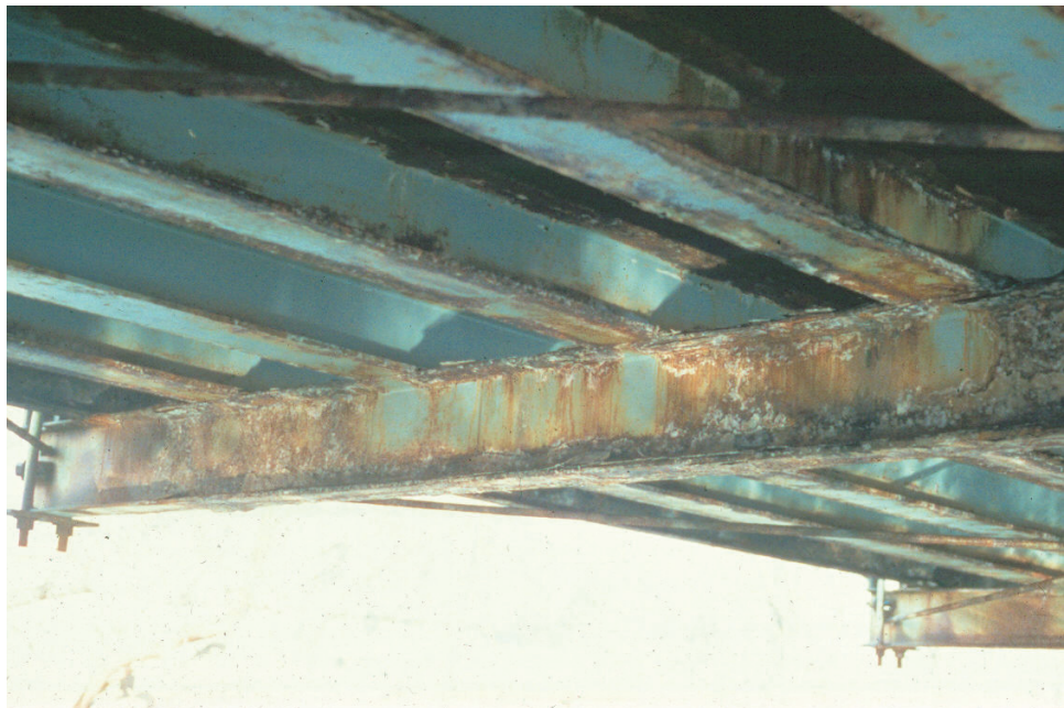
Figure 8.6.56 Corroded Floorbeams and Stringers
