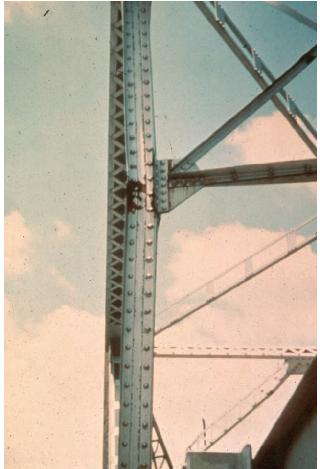
Figure 8.6.51 Collision Damage to Vertical Member
