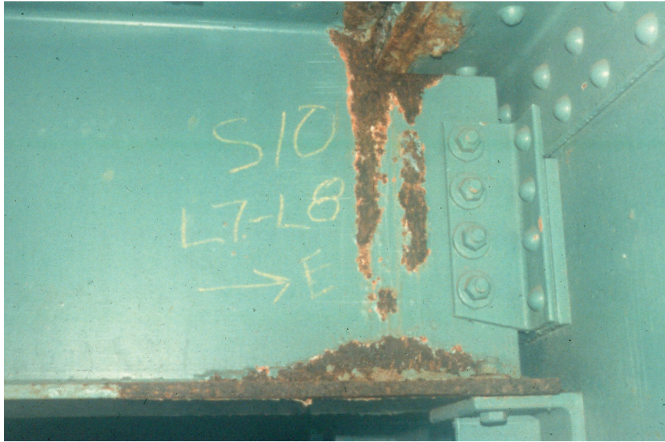
Figure 8.6.55 Corroded Stringer Connection
