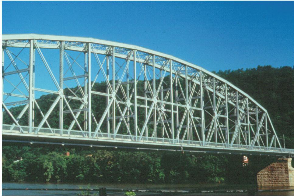
Figure 8.6.32 A Pennsylvania Truss, a Subdivided Pratt Truss with a Camel Back Top Chord
